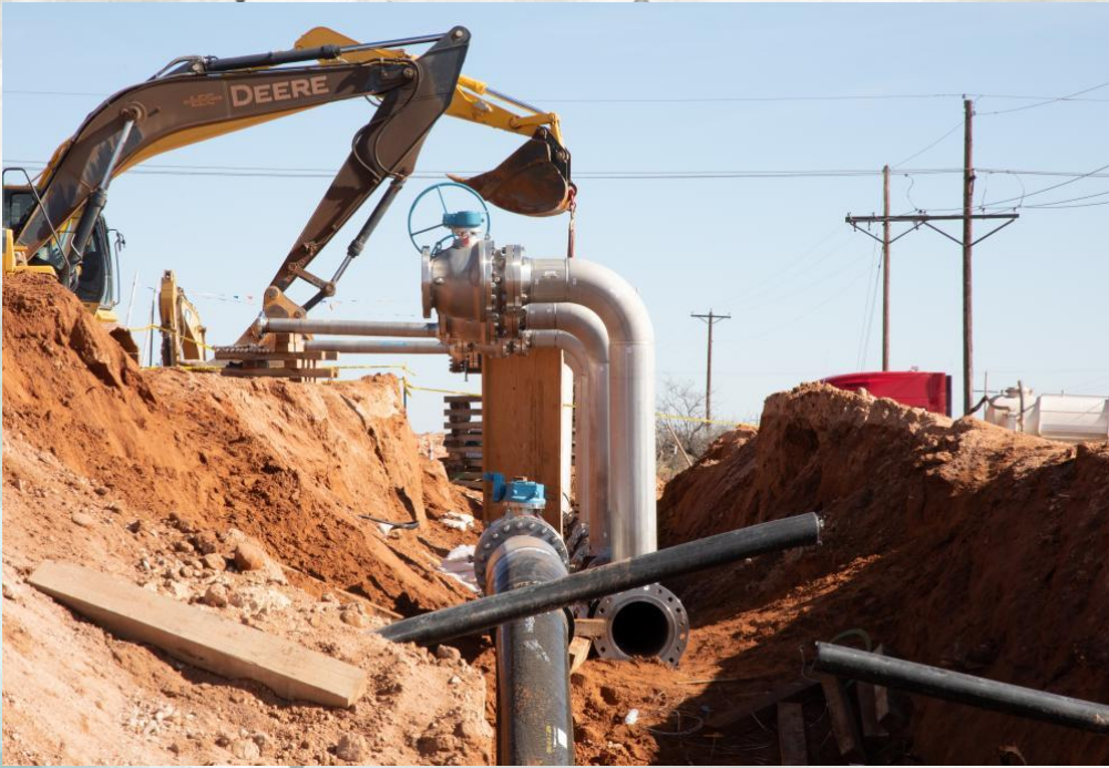
Construction on Goodnight Midstream's 45-mile Llano trans-basin gathering system, located in Lea County, N.M., was recently completed. The pipeline services long-term commitments from large producers with plans for expansion this year. (Source: Goodnight Midstream)
