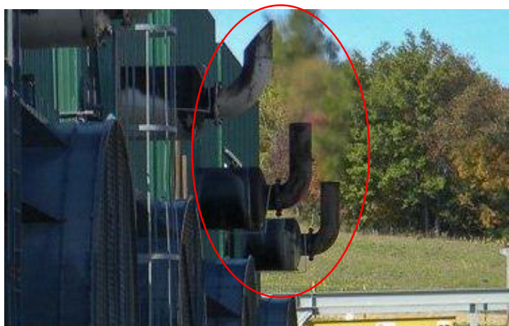
Waste Heat from Compressor Engines
