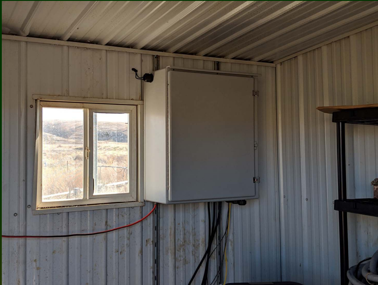
Data acquisition and control box with cellular communications
