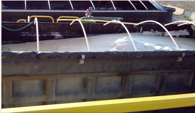
Ox trailer full of dewatered salts from treatment of flue gas desulfurization water at a midwestern power plant. These solids passed paint filtered and disposed of in an onsite landfill.
