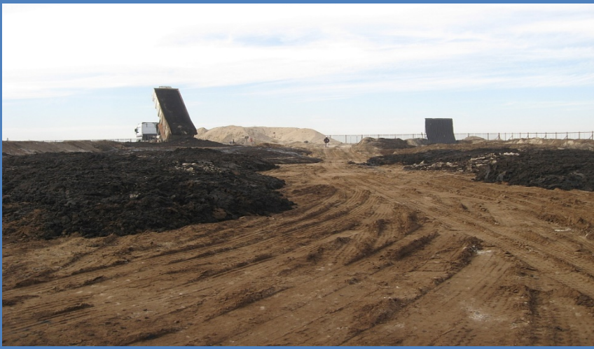
Sludge & Oil Holding Pit
