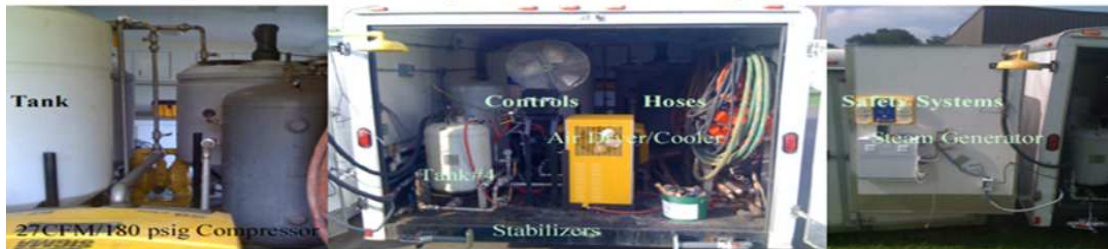
Feed Systems, Safety Systems, Compressed Gas Systems All piping Welded Stainless Steel Floors Coated in Chemical Resistant RinoLining
