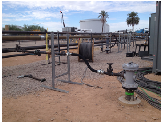
Steam Injection Well
