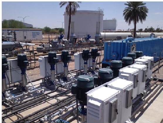
Eductor Pump skids
