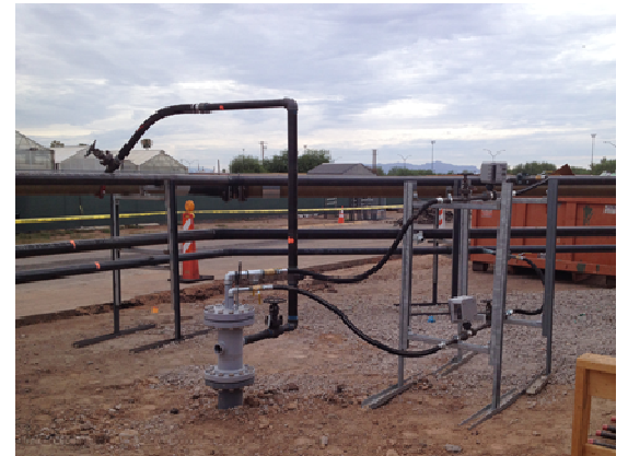
Multi-Phase Extraction Well
