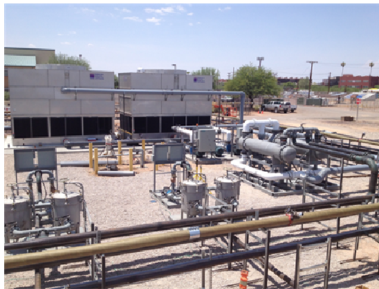
Bag Filters/ Heat Exchangers/ Cooling Towers
