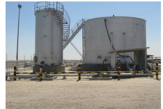
Oil Recovery Plant
