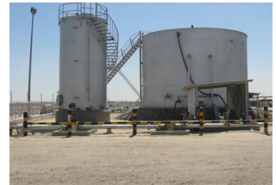
Oil Recovery Plant
