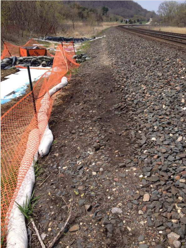
Visual surface staining
