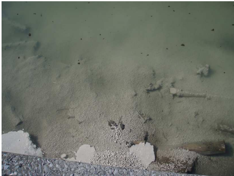
Below and Right: View of AquaGate+Organoclay Being Applied & Close up View in Place
