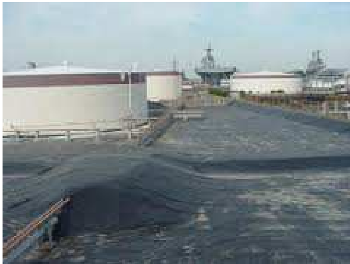
Pipe Penetrations as Containment Failure Point in Berm/Dike
