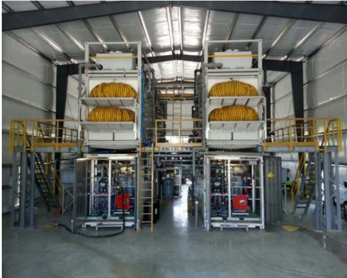
630 bbl/day Containerized and Modular Plant
