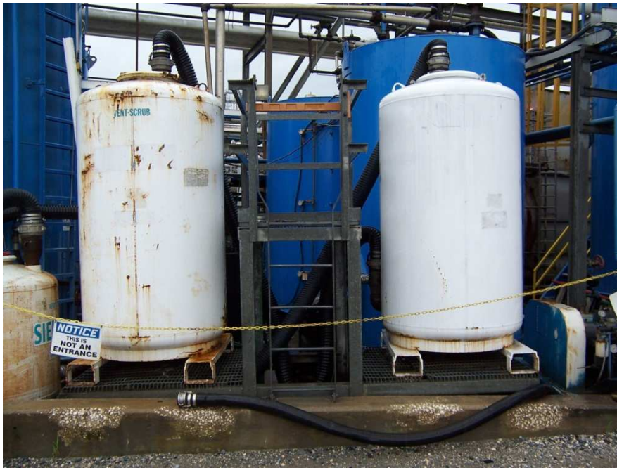
Existing Carbon System
