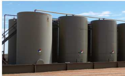
Storage vessels at an oil and gas production facility.
