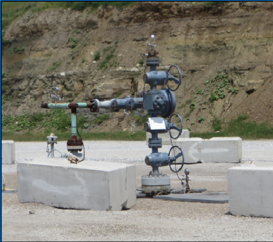
Wellhead in visible light
