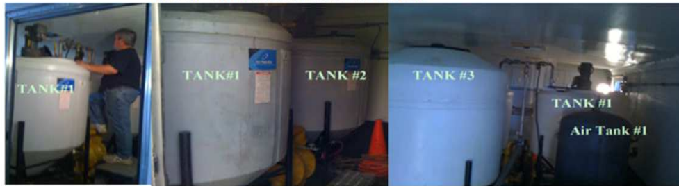
Injection Feed Tank – Configuration
