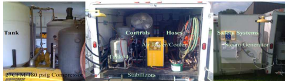
Feed Systems, Safety Systems, Compressed Gas Systems All piping Welded Stainless Steel Floors Coated in Chemical Resistant RinoLining
