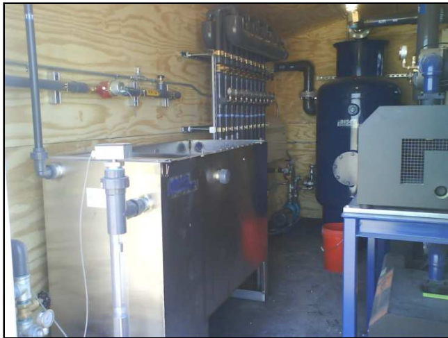
Internal Components of DPE Shed
