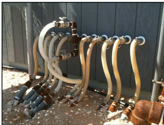
Exterior DPE Shed Manifold
