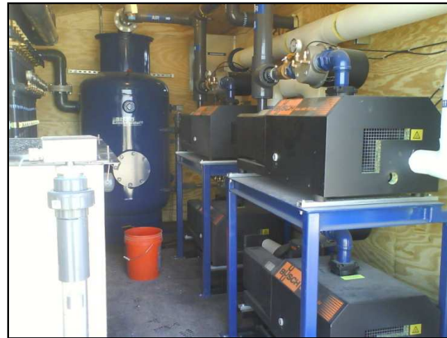
Internal Components of DPE Shed
