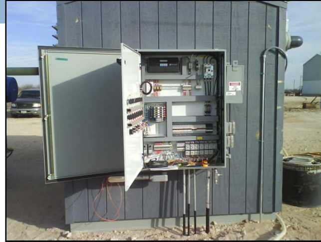
DPE Shed Controller and PLC
