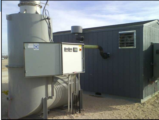
ThermOx Unit and DPE Shed
