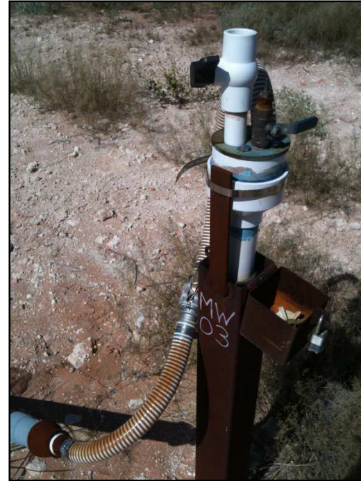
Extraction Well, Wellhead, and Piping
